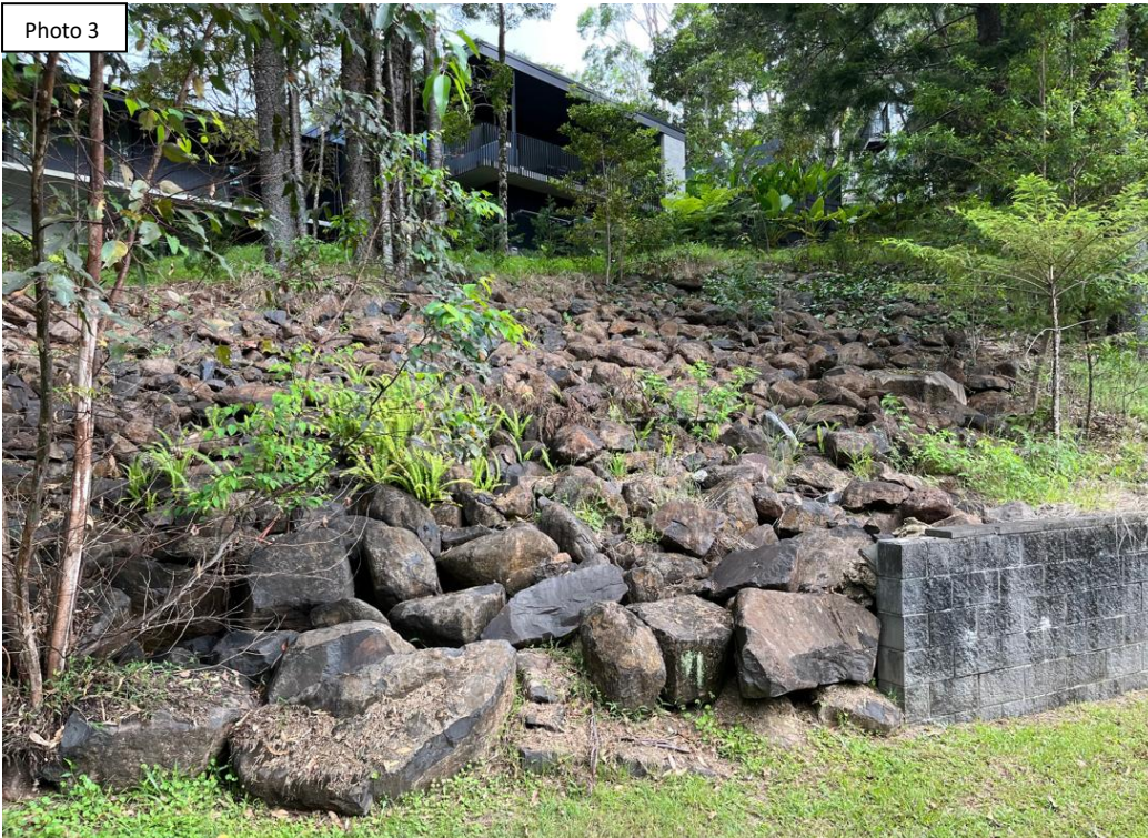
Photo 3 showing the rock retaining wall which is located along Hayters Drive on front of No 14/31.
