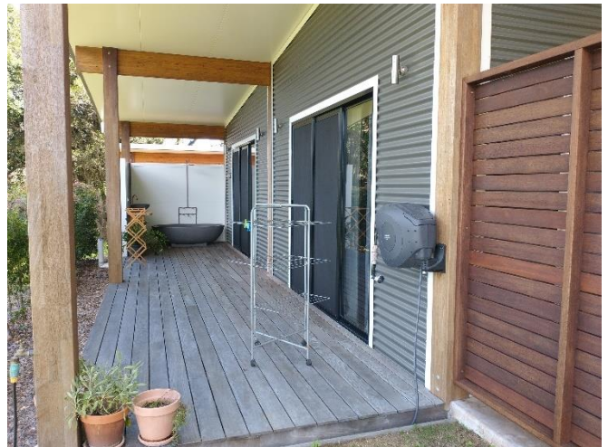
Photo 4 – verandah along eastern wall of dwelling. Vanity next to bath not shown on plans (see Note)
